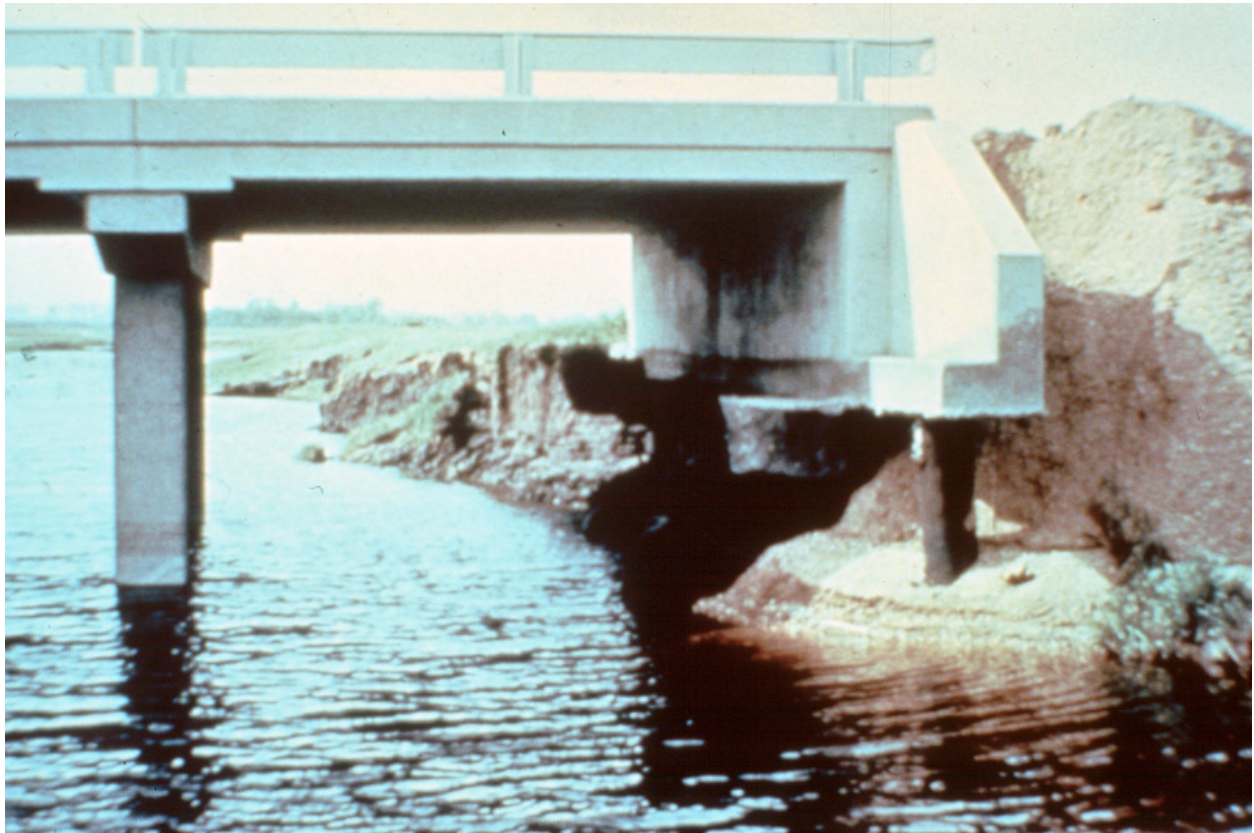
Figure 14.D-A — SCOUR OF BRIDGE ABUTMENT AND APPROACH EMBANKMENT
