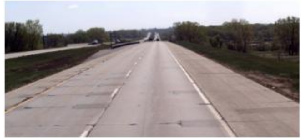
Photo of Existing Pavement Showing Repairs and Spalling
