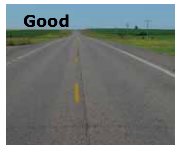
Good Visible, light traffic wear, with limited, narrow crosswise and lengthwise cracking
