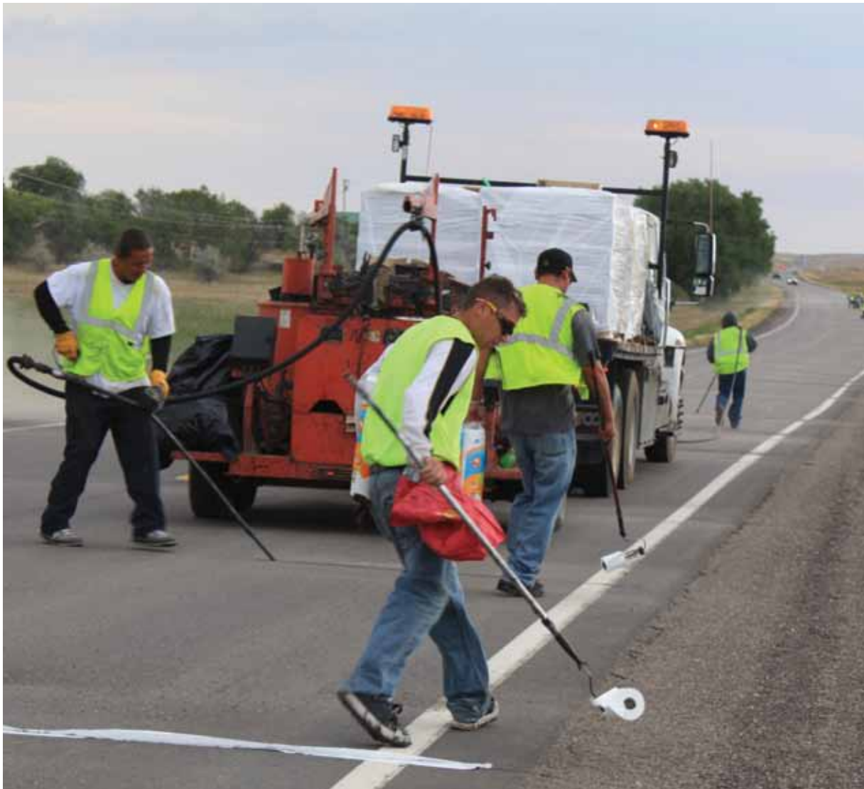
A contractor crew fills cracks in asphalt concrete pavement with hot asphalt crack sealant and rolls tissue across the seal on state Highway 34 in western South Dakota. Up ahead, workers rout cracks and then blow out loose material. This preliminary work helps ensure a long-lasting seal. Crack sealing is one of the most basic and critical types of road maintenance, preventing water from infiltrating the road foundation and thereby lengthening its service life. Crack-sealing projects play an important role in the South Dakota Department of Transportation's effort to preserve existing infrastructure and provide a smooth ride.
