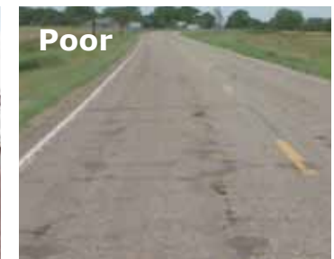
Poor Deteriorated patching, extensive lengthwise and crosswise cracking, significant rutting
