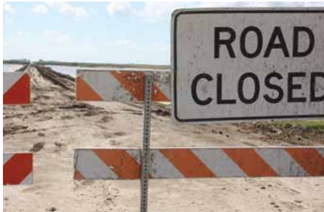
Top: Chunks of South Dakota Highway 44 east of Parkston broke off in 2011 after James River floodwaters undermined the road's foundation. In the background, DOT employees from the Menno shop work on temporary repairs. Bottom: South Dakota Highway 10 was closed for most of the summer of 2010 as clay was hauled in to raise the grade.
