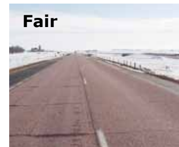
Fair Slight rutting, increasing aggregate loss, increasing width and extent of cracks
