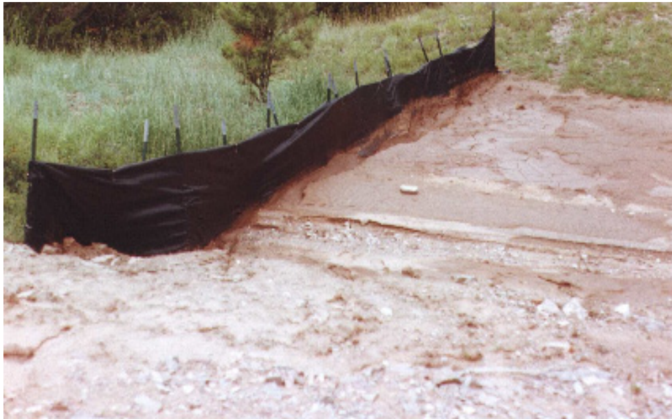
Figure 5.27 Silt fence performing its intended function
