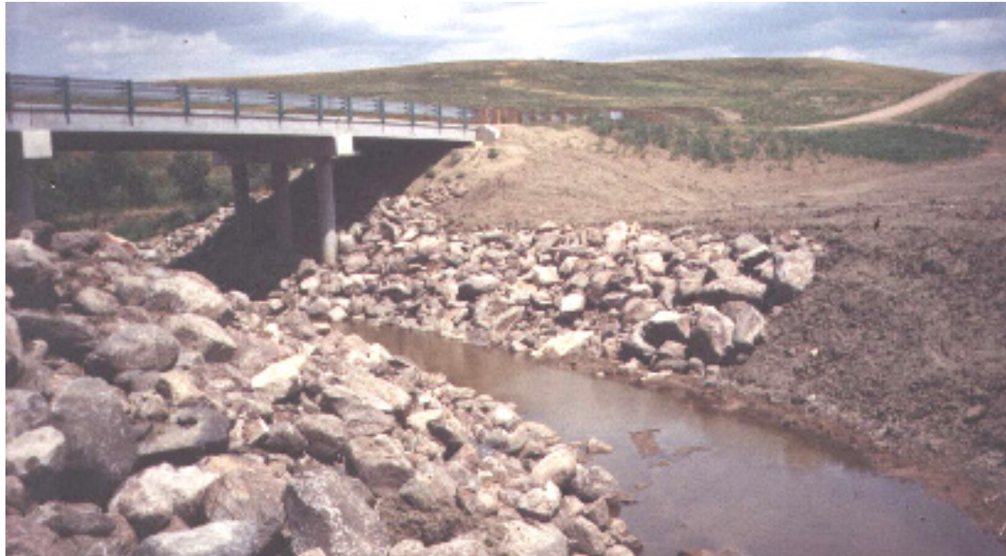
Figure 5.19 Example of RipRap used along channel and bridge berm.
