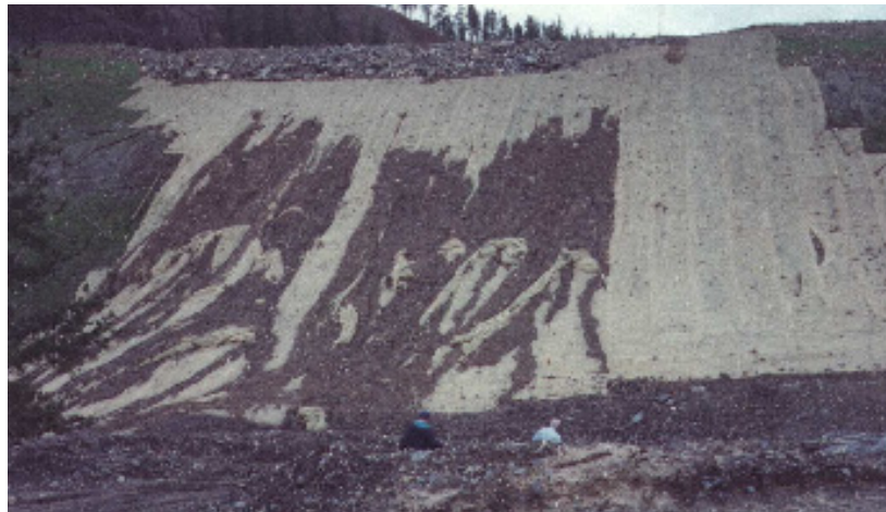
Figure 5.8 Excelsior Blanket Failure.
