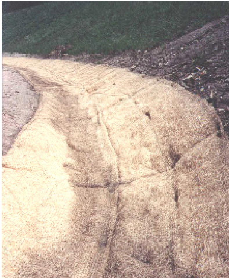
Figure 5.7 Incorrect Placement of Erosion Control Blanket
