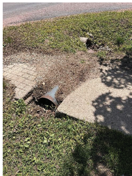
Debris impeding drainage
