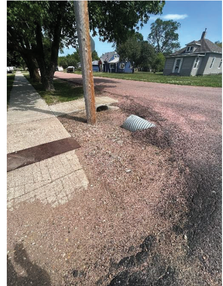
Debris impeding drainage
