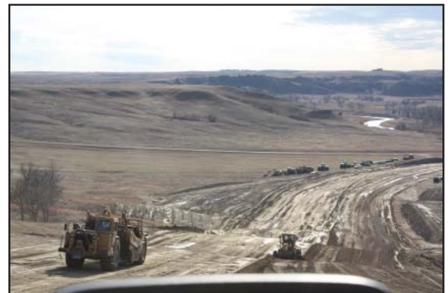
Earth Moving Equipment in 2011. Highway 65 construction project north of Isabel. The more things change, the more they stay the same.
