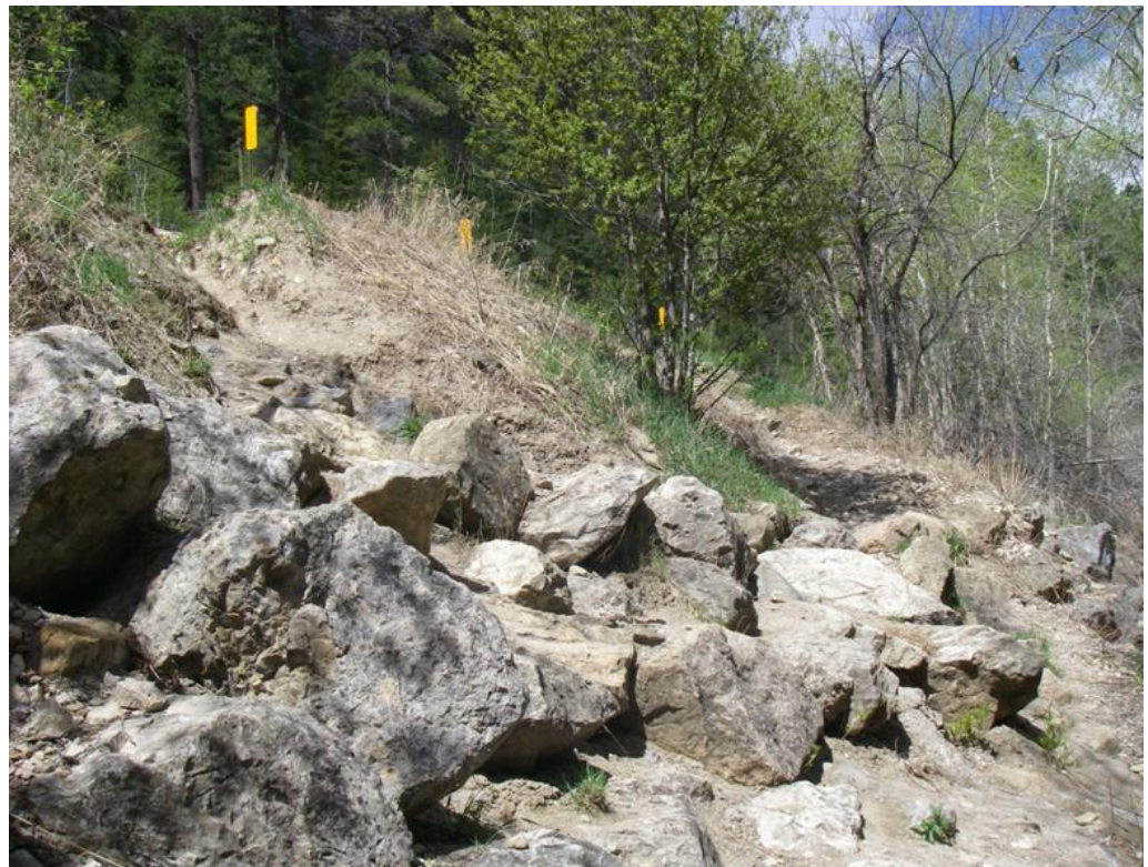
Photo illustrating erosion along the steep slope below U.S. Highway 14A at the Bridal Veil Falls Site
