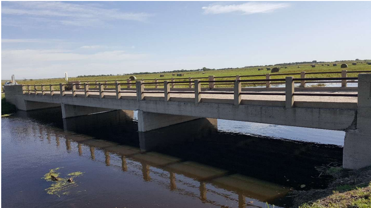
Bridge on 310 th Avenue; note the deteriorated concrete.
