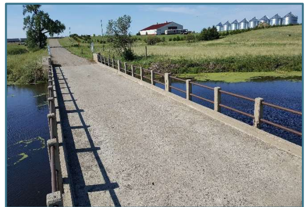
This bridge east of Blunt was constructed in 1934, is currently posted for load restriction, and has a sufficiency rating of 26.9.
