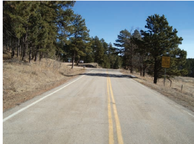
FIGURE 11 – Vertical Curvature on Silver Mountain Road with Boulder Hill Road in the Background (Camera Facing Northeast)
