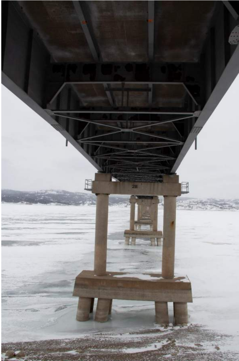
View below easternmost spans of the Platte-Winner Bridge showing the floor system of floor beams, stringers, underside of deck, and the supporting eight-pile pier, view facing west.
