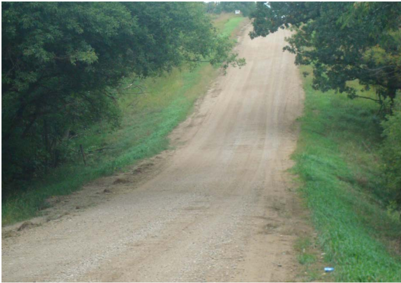
456 th Avenue With Steep Slopes and Recent Shoulder Maintenance
