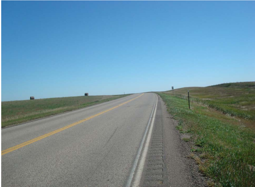
US Highway 12 (MP 116.3) Reverse Superelevation
