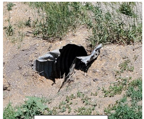
Damaged pipe culvert
