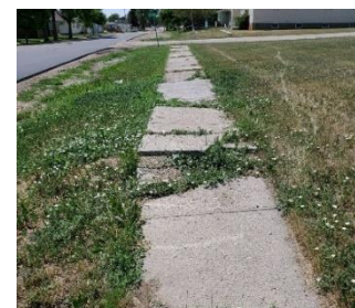
Poor Sidewalk Quality
