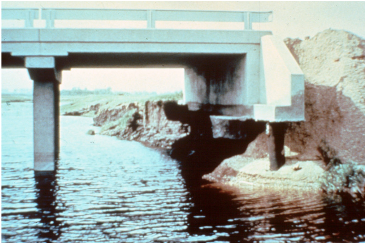
Figure 14.D-A — SCOUR OF BRIDGE ABUTMENT AND APPROACH EMBANKMENT
