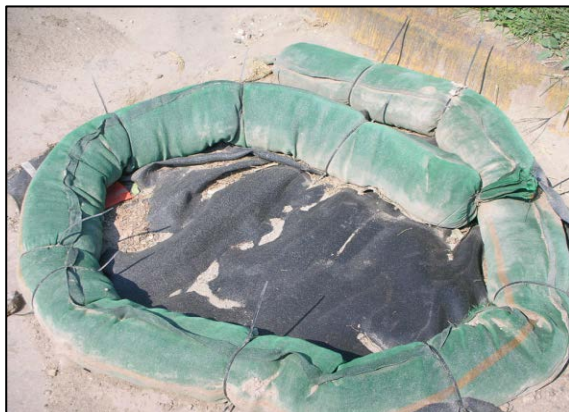
FAA Stormwater Management at the Capital Avenue Reconstruction Project in Pierre 2009 – Inlet protection. (Dale Healey, SDDENR)
