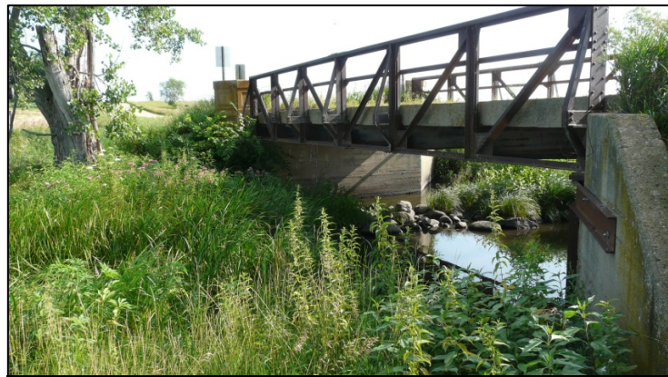
Environmental resources in the project area are identified by desktop review or site inspection. (SDDOT)
