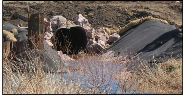
Stream diversion on a Turner County project. Culverts with a 60-inch diameter were used to divert the creek around the project area. (SDDOT)
