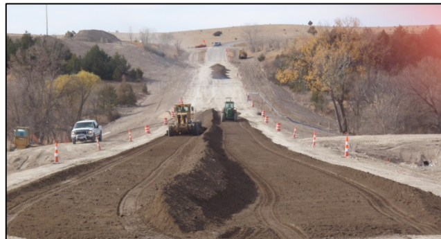
Work limits that are minimize during final design can reduce the effects on environmental resources and demonstrates good faith efforts in minimizing environmental impacts. (SDDOT Staff)
