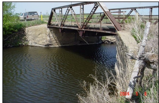
Structure field inspection to determine if aquatic species may be affected by replacement. (SDDOT)
