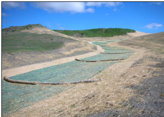
Stormwater Management at the Pierre Landfill Cap Project 2009 – straw wattles/mulch/turf reinforcement mat. (SDDENR)
