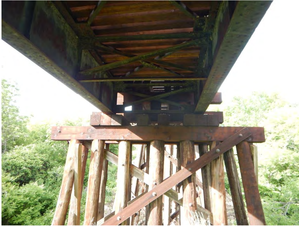
Photo 1. Railroad bridge facing northeast; no NLEB roosting habitat - spaces not sealed from weather
