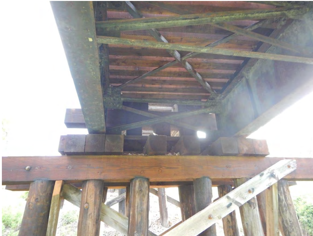
Photo 2. Railroad bridge facing southwest; no NLEB roosting habitat – spaces not sealed from weather
