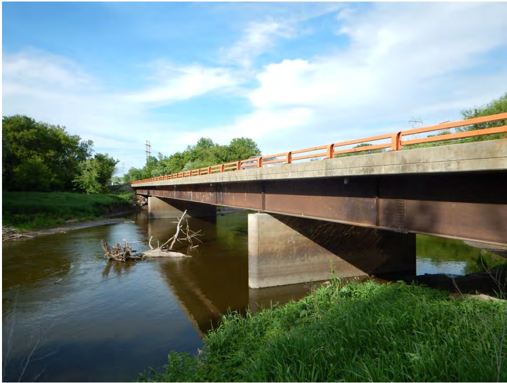
Photo 3. Timberline Ave. bridge over Big Sioux River facing northeast; no NLEB habitat, no vertical cracks
