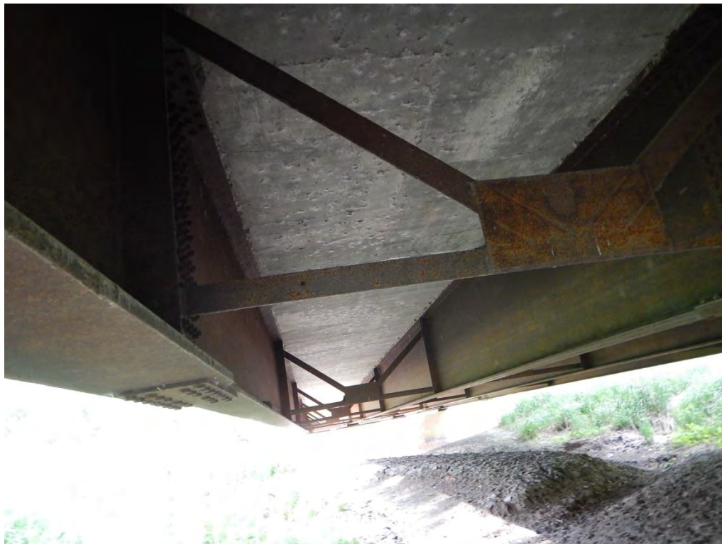
Photo 4. Timberline Ave. bridge over Big Sioux River facing east; no NLEB habitat, no vertical cracks
