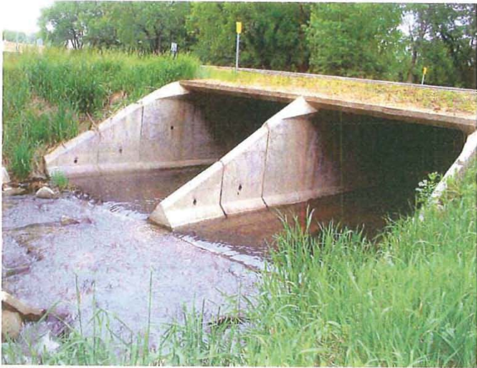
Figure 1: Outlet of box
