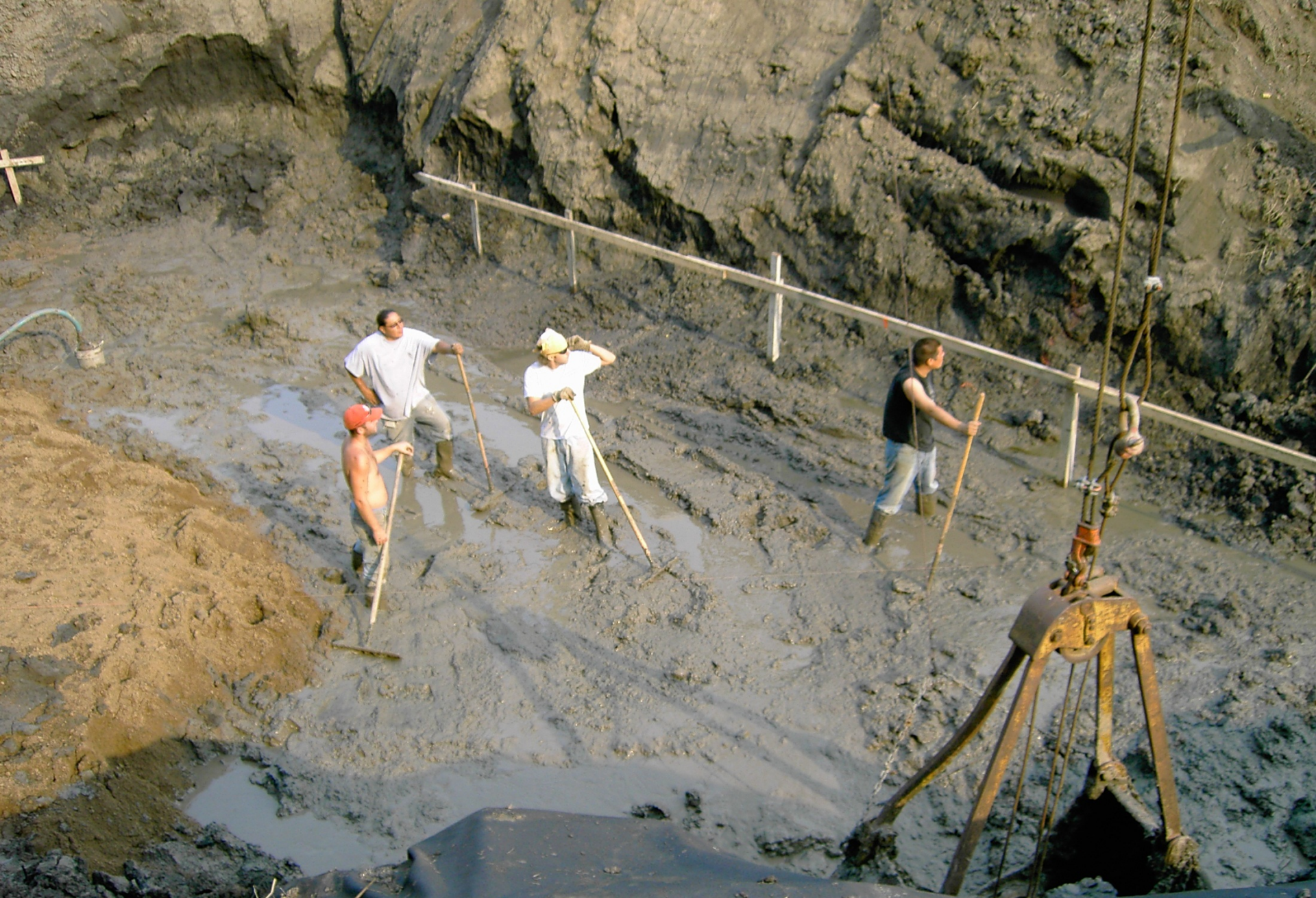
Box Culvert Undercut
