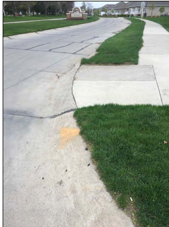
A rolled-curb transition no longer complies with the ADA.
